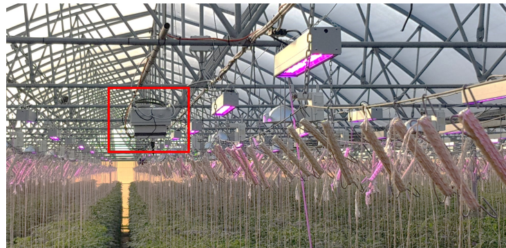
Figure 5. Sensors installed inside the greenhouse with the electrical cabinet containing the data monitoring unit hanged to the greenhouse cover.
