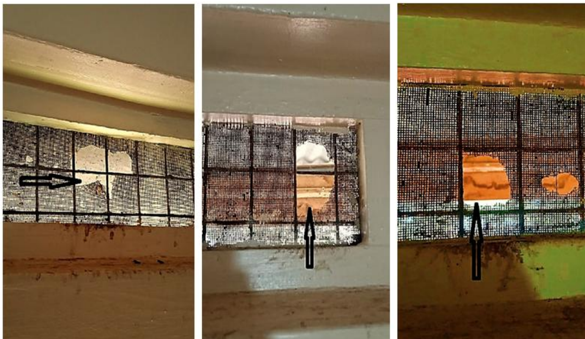
Fig. 10. Representative image for damaged ventilation wire meshes found in one of the students' on-campus residences at IUIU
